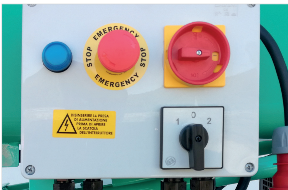
Tph Machine Control Panel
