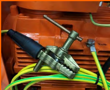
Earth Cable with Clamp.
