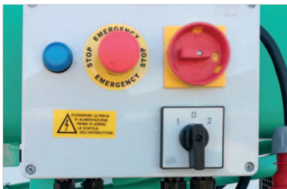
Tph Machine Control Panel
