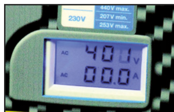
Volts and amps meter control display.
