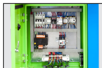
Control panel box.
