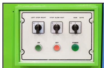
Complete command centre.
