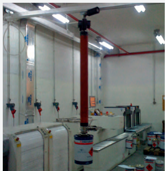
ATEX zone 1 installation, ejector driven VM120, standard suction foot art nr 630215.
